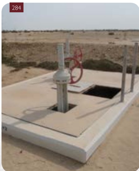
Valve pit in Ras Laffan
